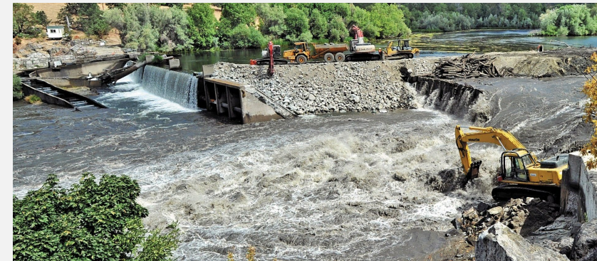
Removal of Gold Ray Dam on the Rogue River, Jackson County, 2010, Oregon
